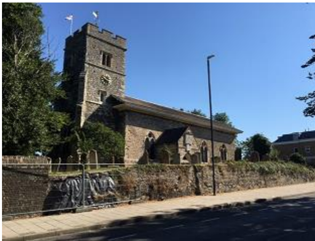
Flint section of the wall along East Milton Road, including the collapsed section
